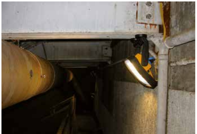
Tunnel illumination, supply tunnel
