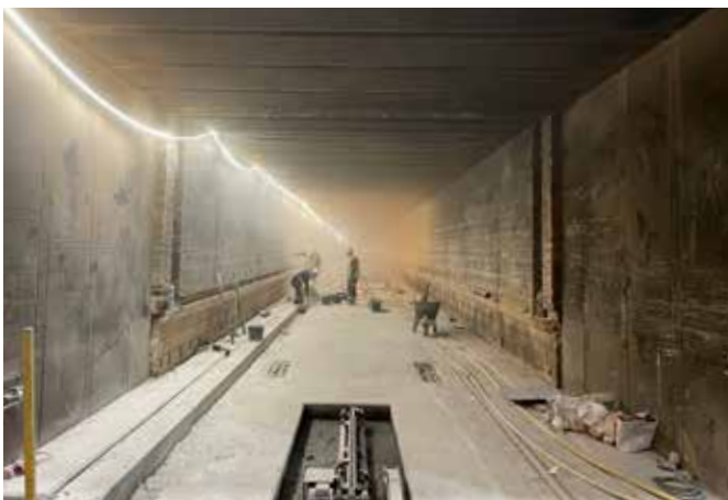
Maintenance lighting, drying oven
