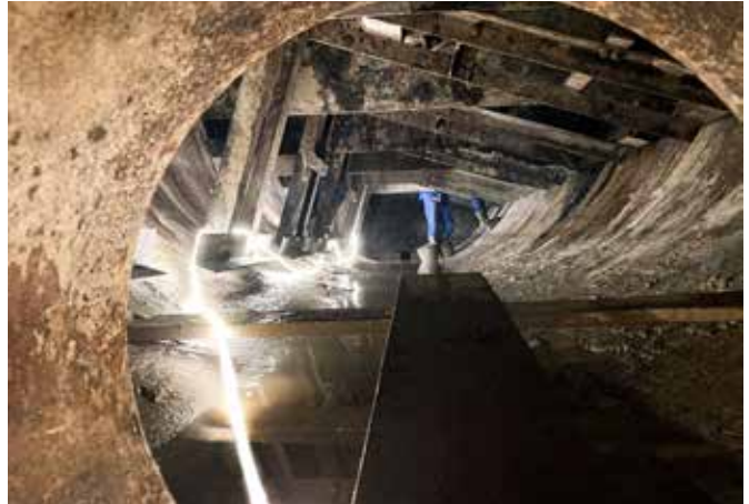
Maintenance lighting, silo
