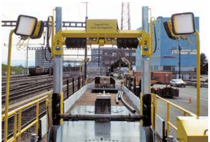
Stationary lighting, maintenance system
