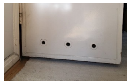
Holes for transfer air
