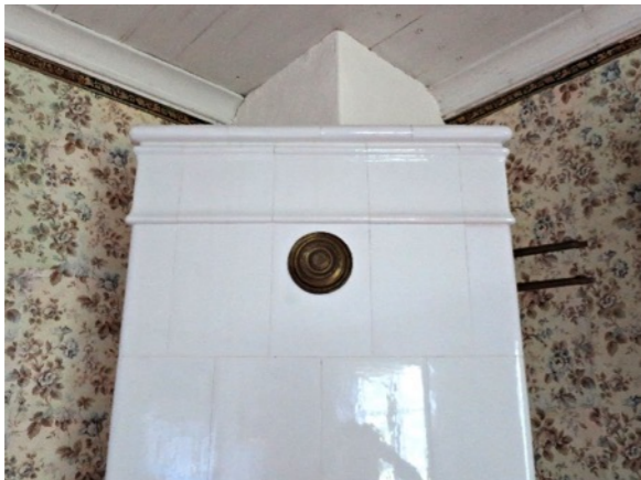
Exhaust vent in a masonry stove
