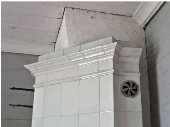
Exhaust vent in a masonry stove
