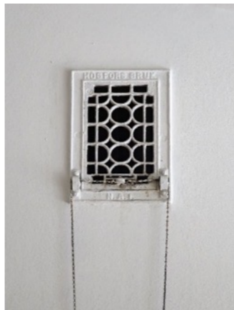
Cast iron vent for exhaust air
