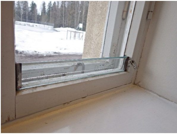
Supply air taken in between the panes. Photos: Anu Laurila
