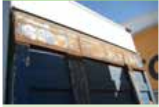
A lifting mechanism with repair signs but in full operational order.
