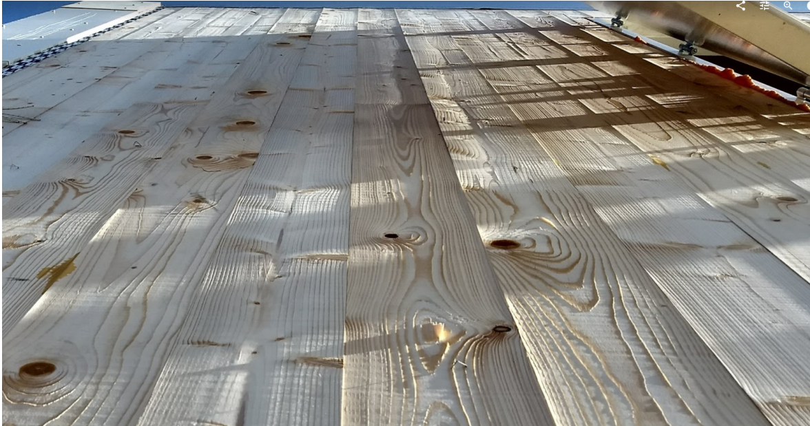
Figure 3.1. Visible deformation of boards exposed to weather conditions. Photo is taken six months after the test
