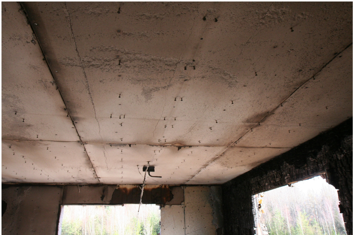
Figure 4.13. The third layer of gypsum fell off during extinguishing
